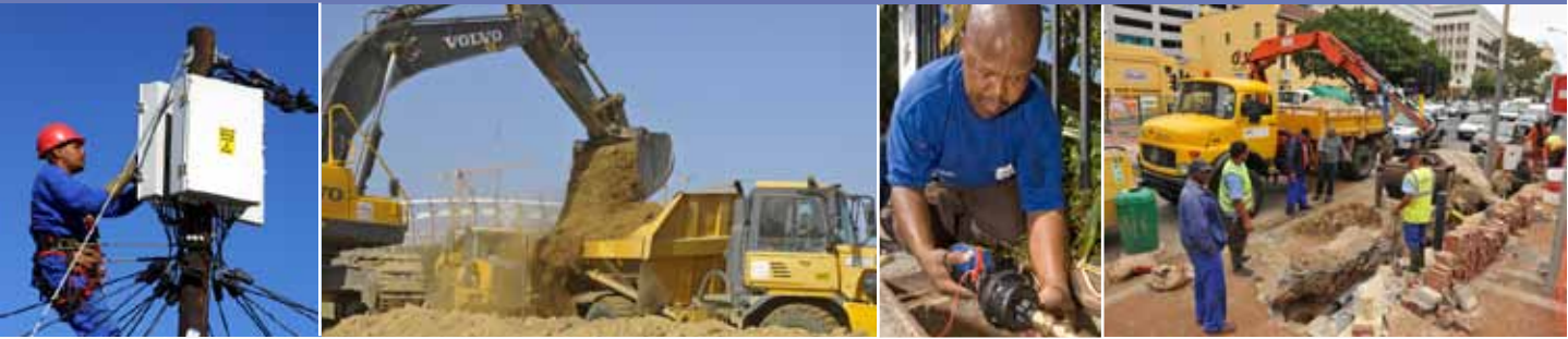
Tariff increases are necessary to address operating requirements, maintenance, sustainability and to provide new infrastructure
